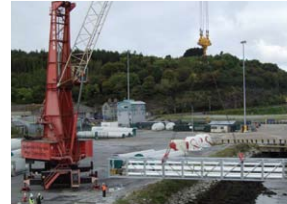
G1 crane placing the pipe bridge across the back of No. 3 jetty as part of the new AFSC terminal project.
